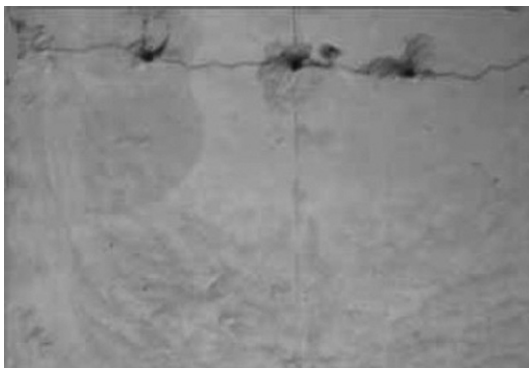
Fig. 19. Image of the subway inner wall including leakage, spall, and other forms of damage.
